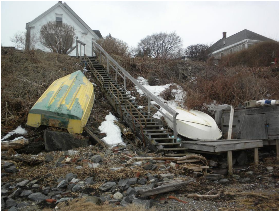
Stairs to be replaced - Photograph taken march 28, 2015
