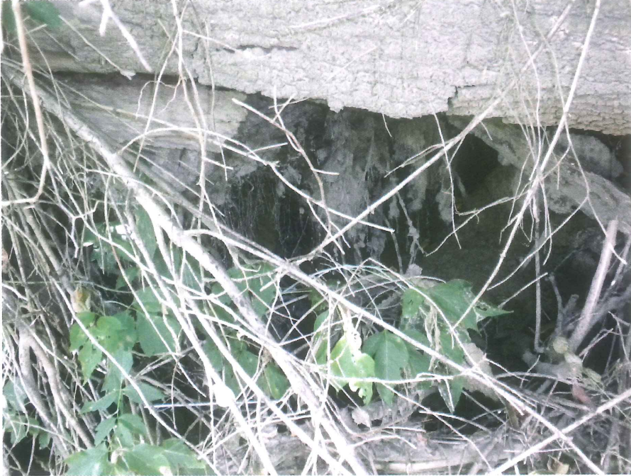
Photograph # 5 Slope slump where trees have uprooted.
