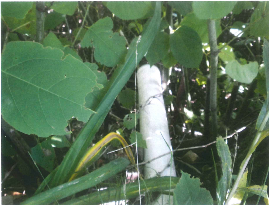
Photograph #8 drain pipe outlet on the embankment. The drain is connected to the roof gutter system.
