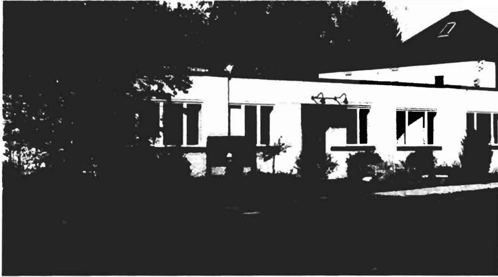
Front of building showing building mounted sign being replaced and free-standing sign being removed
