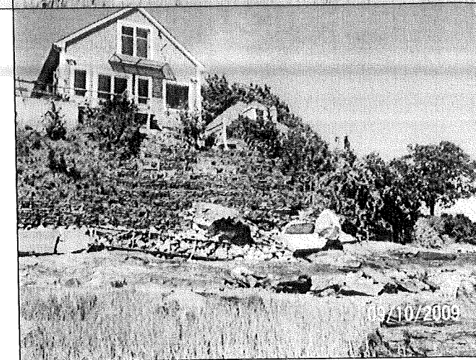
② FRONT VIEW OF LOBSTER TRAP GABIONS, EXISTING RETAINING WALL AND DEBRIS AT BASE OF EMBANKMENT.
