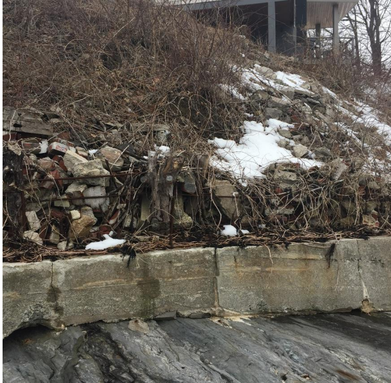
Watson Street Property, existing deteriorated seawall at the toe of slope
