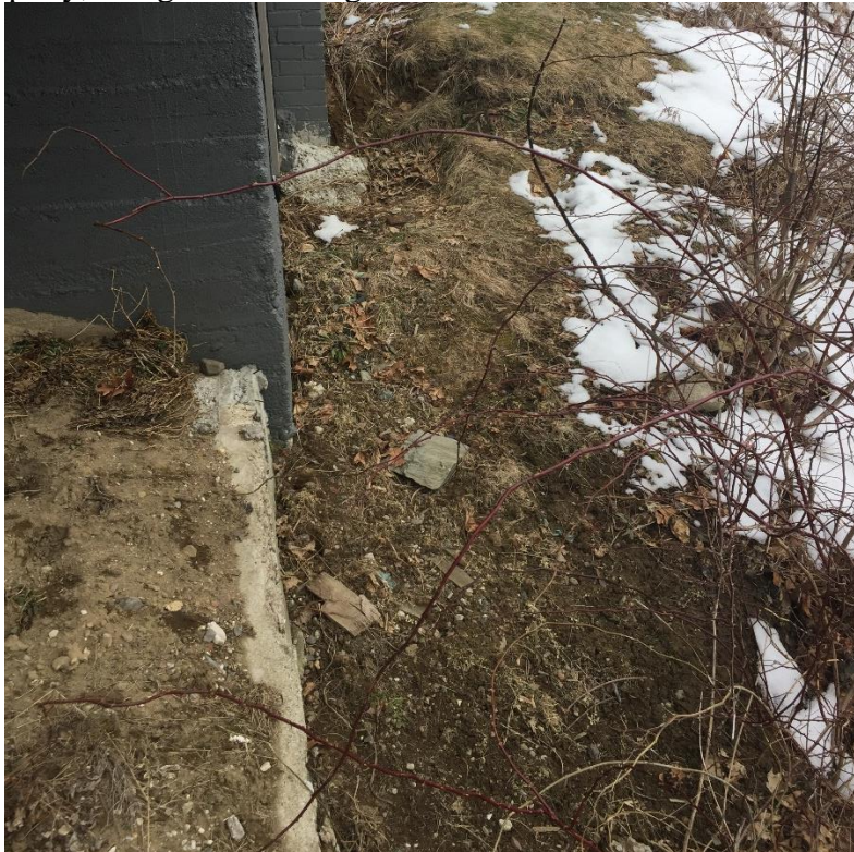
Watson Street Property, Erosion near foundation of existing residence near top of slope.
