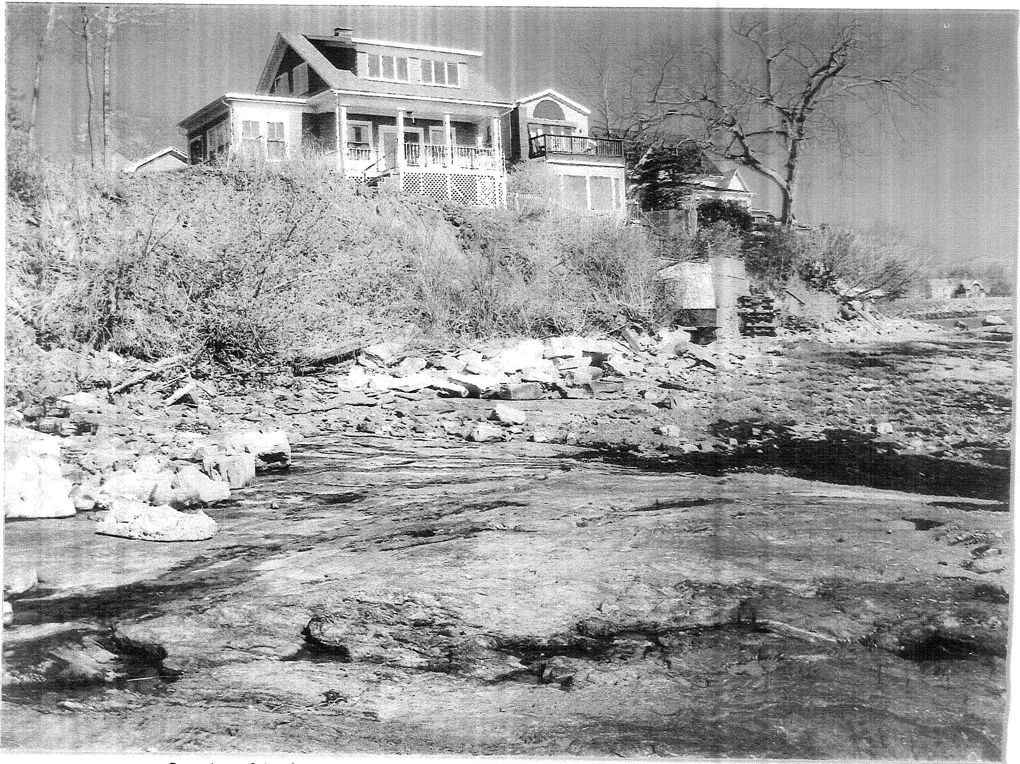
Overview of 6 Island Street, Portland property with failed retaining wall and eroded bank
