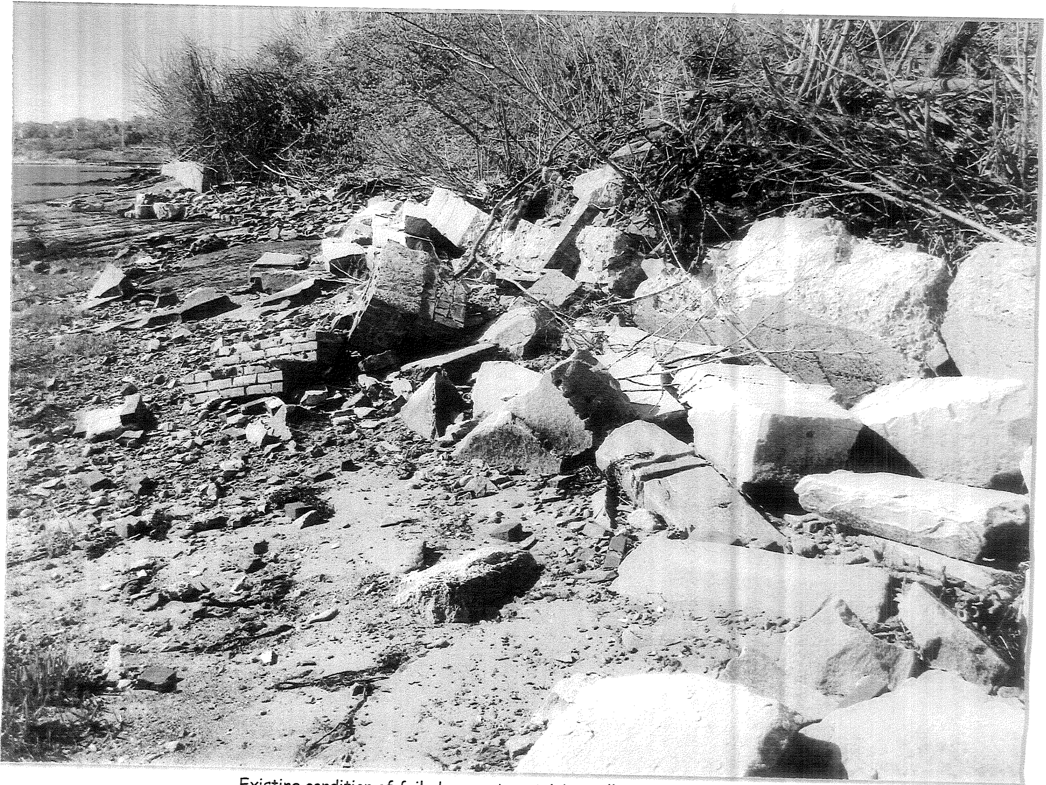
Existing condition of failed concrete retaining wall and abutting property.
