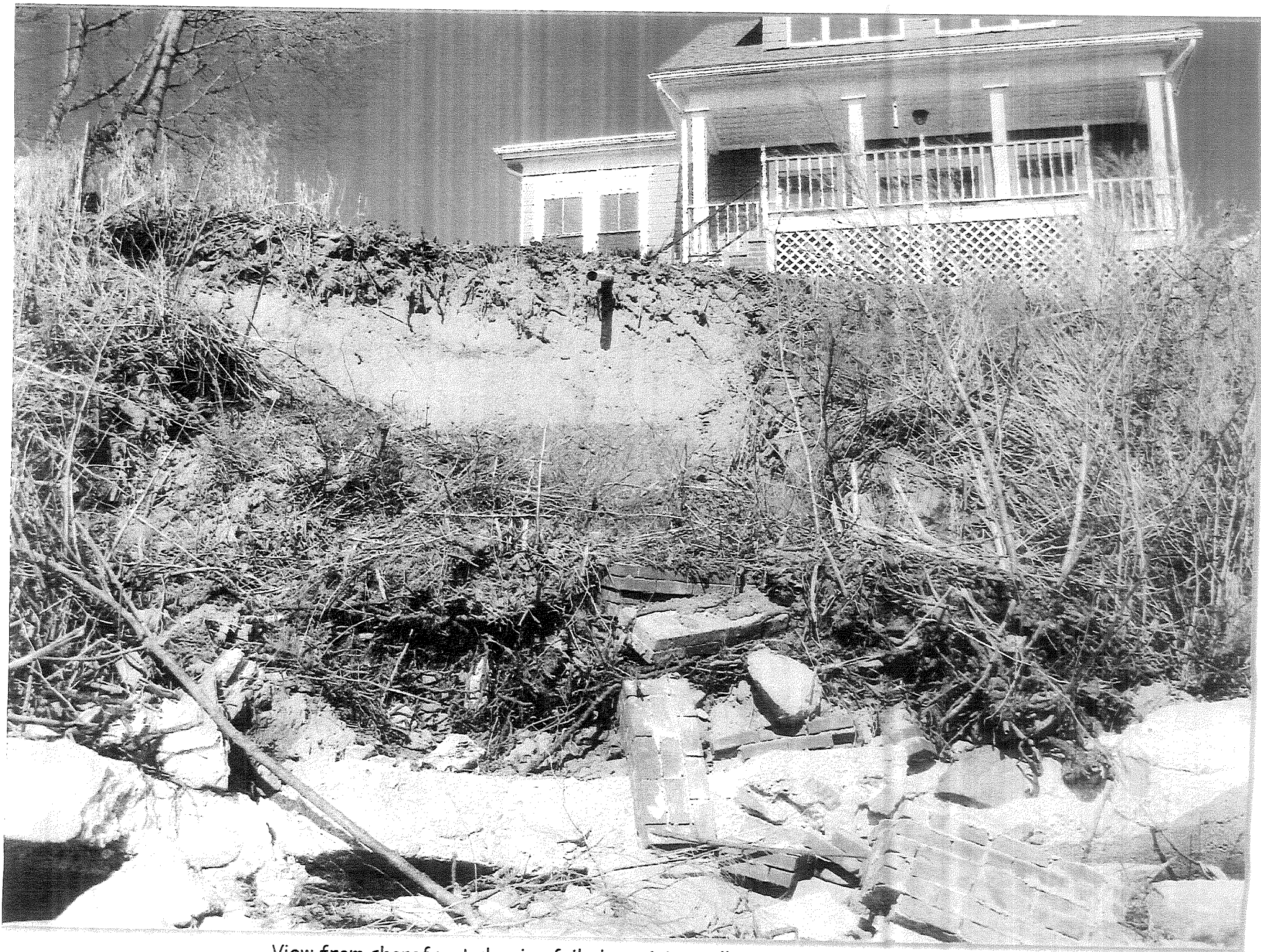
View from shorefront showing failed retaining wall and eroded /slumped bank.
