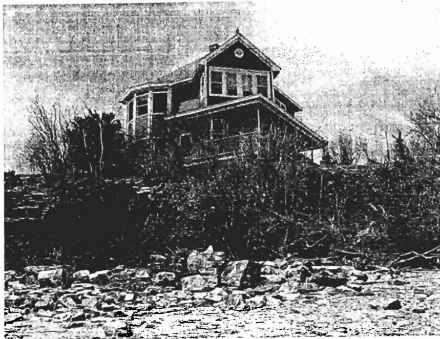
Eroded bank North of wall section. Top of eroded bank is ~12 feet from house.
