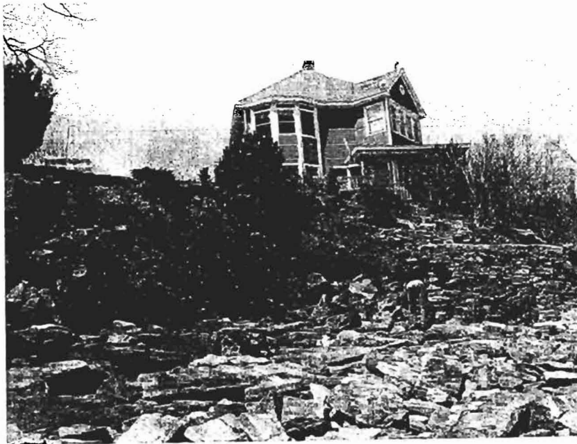
Eroded bank with remaining section of wall showing. Note ledge base.
