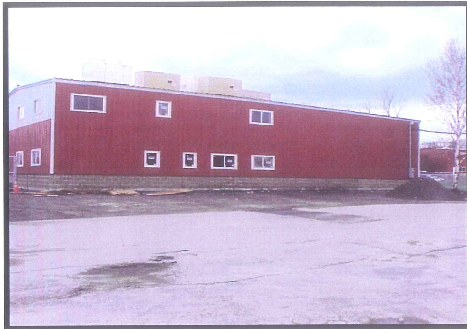
PHOTO 4B: View of north side of building with new siding and windows.
