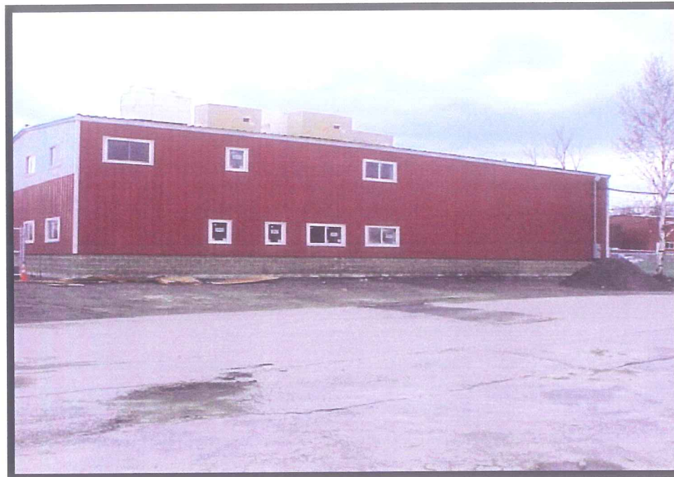
PHOTO 4B: View of north side of building with new siding and windows.
