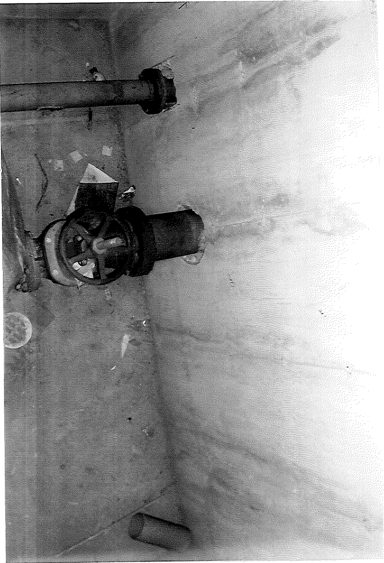
This is looking down - it's about 10 to 12 feet down. There is no ladder or stairs.
