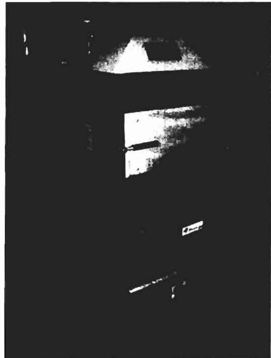
Fig. 5: - overall view of the boiler (with a combustion chamber test door and covered fan)
