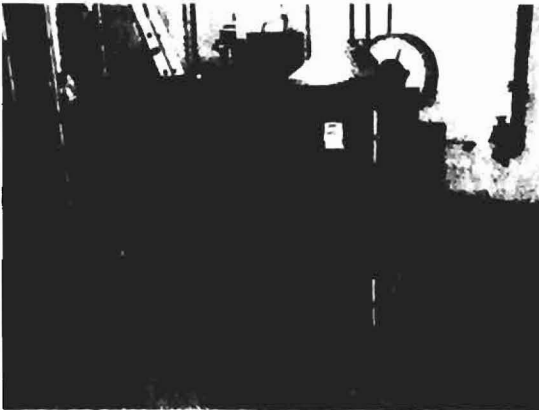
Fig. 2 - overall view of the boiler
