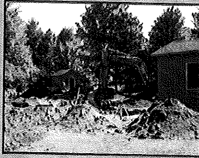
Our excavator will begin digging the pool site to the correct depth and shape.
