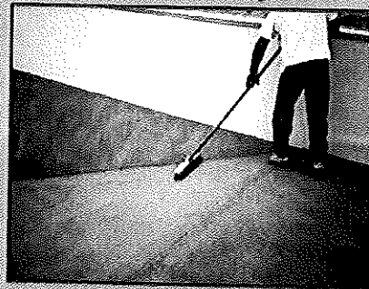
Once the vermiculite has hardened, it is cleaned and prepared for the liner.
