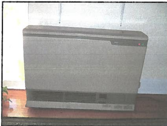
* Monitor heat (Unit 2)
