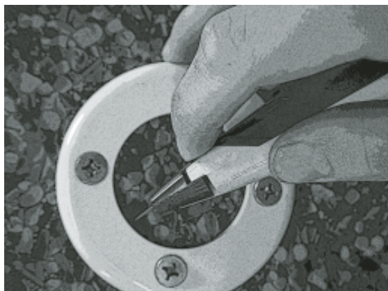
Trim liner from return opening.
