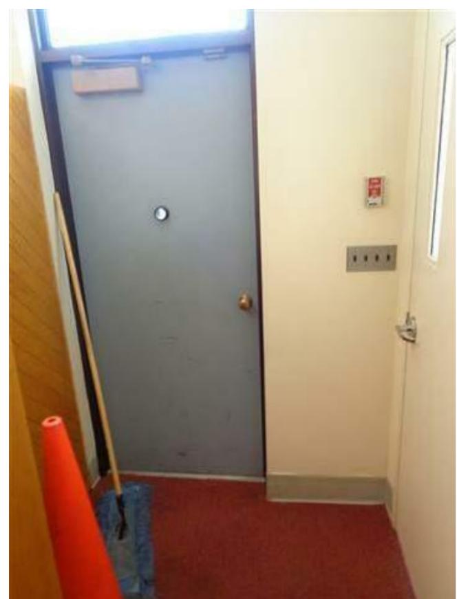
REAR EGRESS DOOR AND FA PULL TO BE MADE COMPLIANT
