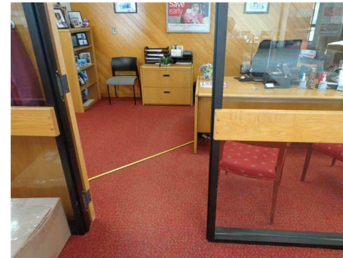
CARPET TO BE REPLACED
