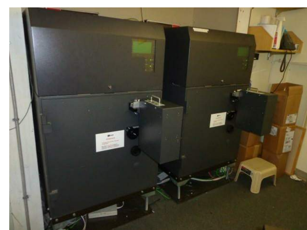
RELOCATE ONE ATM. RELOCATE AND LOWER SECOND ATM TO COMPLY WITH 2010 ADAAG.
