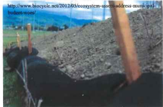
Erosion control socks used to prevent sediment from moving on a slope in California.
