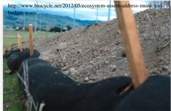
Erosion control socks used to prevent sediment from moving on a slope in California.
