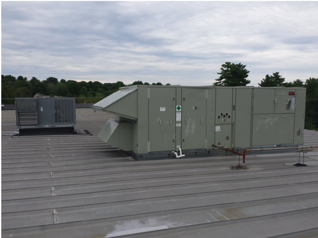
Photo 1: Existing mechanical unit location relative to new mechanical unit.
