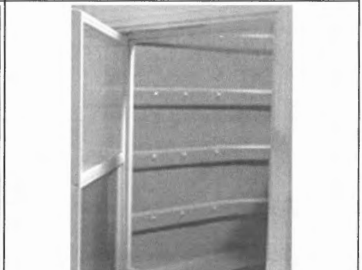
IN FINISHED BASEMENTS, BY LAW, A SECOND MEANS OF EGRESS IS REQUIRED.
