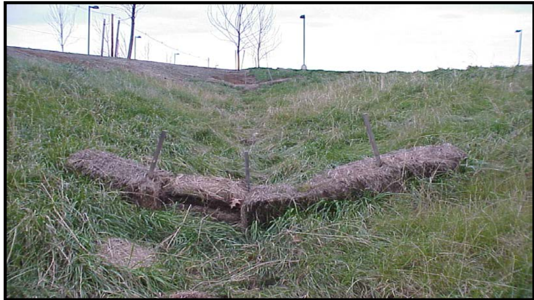
VEGETATED SWALE WITH HAY BALE CHECK DAM TO REDUCE VELOCITIES UNDER CONSTRUCTION
