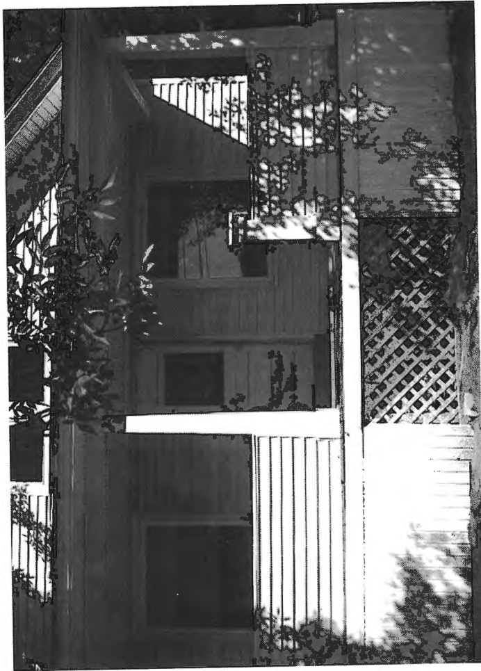
VIEW OF FORMER STAIR AREA (ROTTED)
