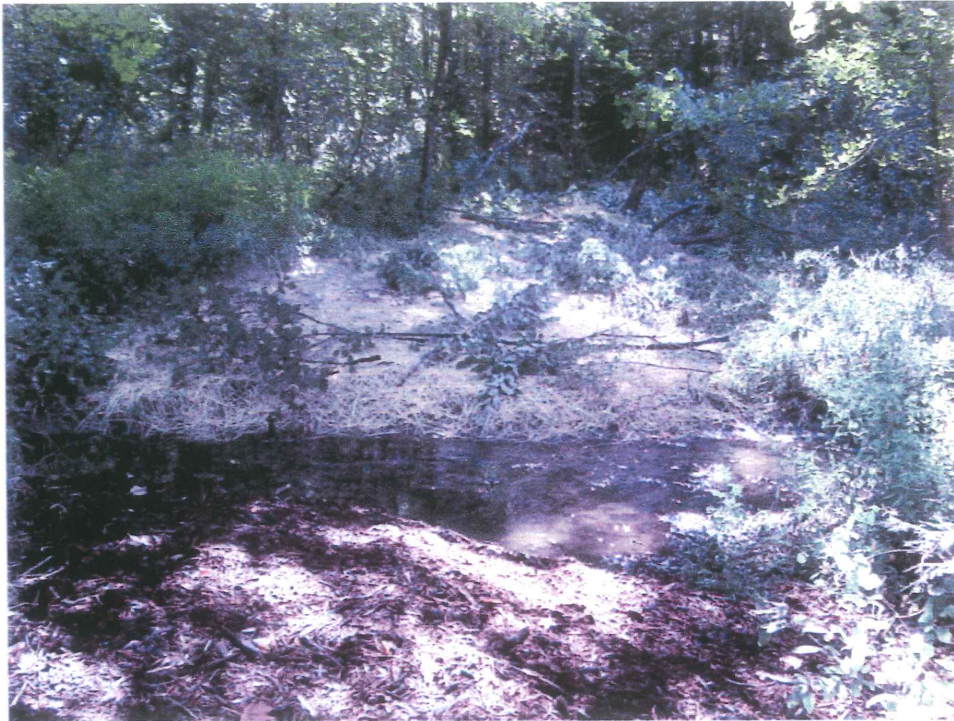
Photograph 3 Eastward view across Capisic Brook where culverts and berm were removed to restore the wetland; now covered with straw mulch to prevent erosion and replanted with wetland shrubs.
