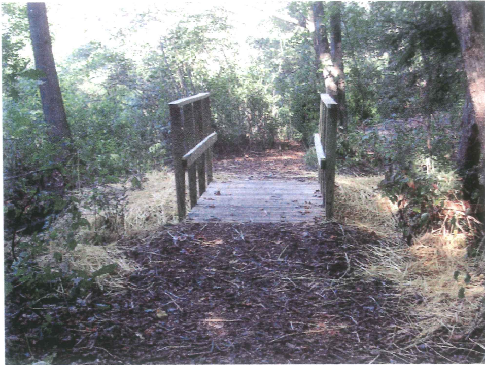
Photograph 1 Northward view along the main trail where culverts were removed at the stream crossing and replaced with a new wooden bridge on granite footings. Both banks of the stream channel were stabilized with straw and planted with wetland shrubs.
