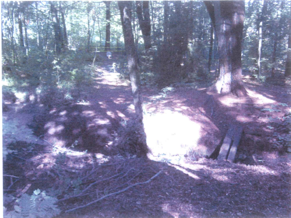
Photograph 5 Westward view of area where the fifth culvert was removed (left side of photo) to relocate the trail out of the wetland that was replanted with a mixture of wetland shrubs.
