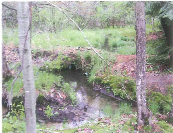
1. Looking southwest at the 10- and 14 inch culvert wetland is in the background.
