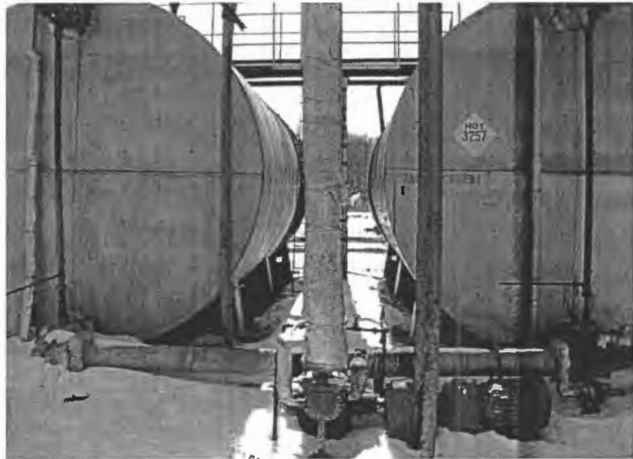
PHOTO 4 Non-ACM pipe & tank insulation
