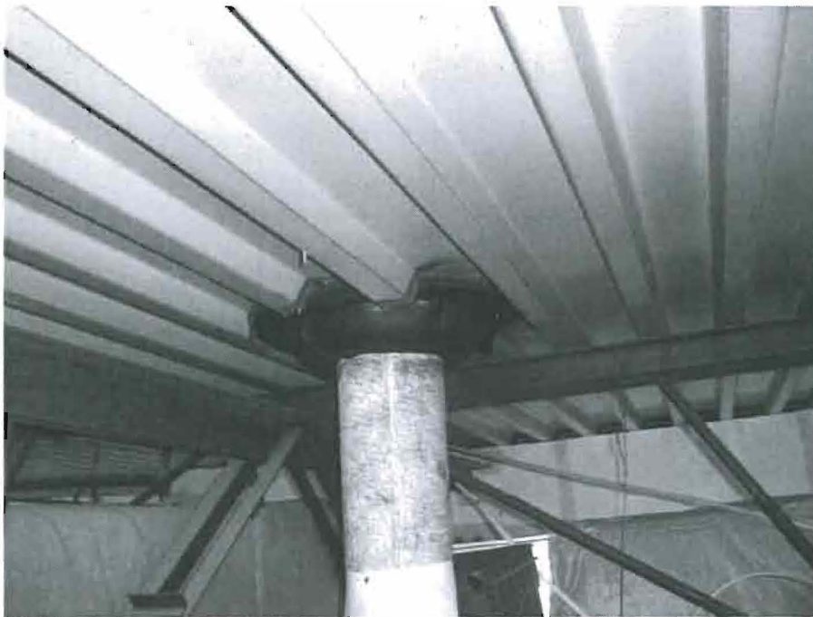
Photo 1: Unreinforced deck penetration at existing roof drain body.
