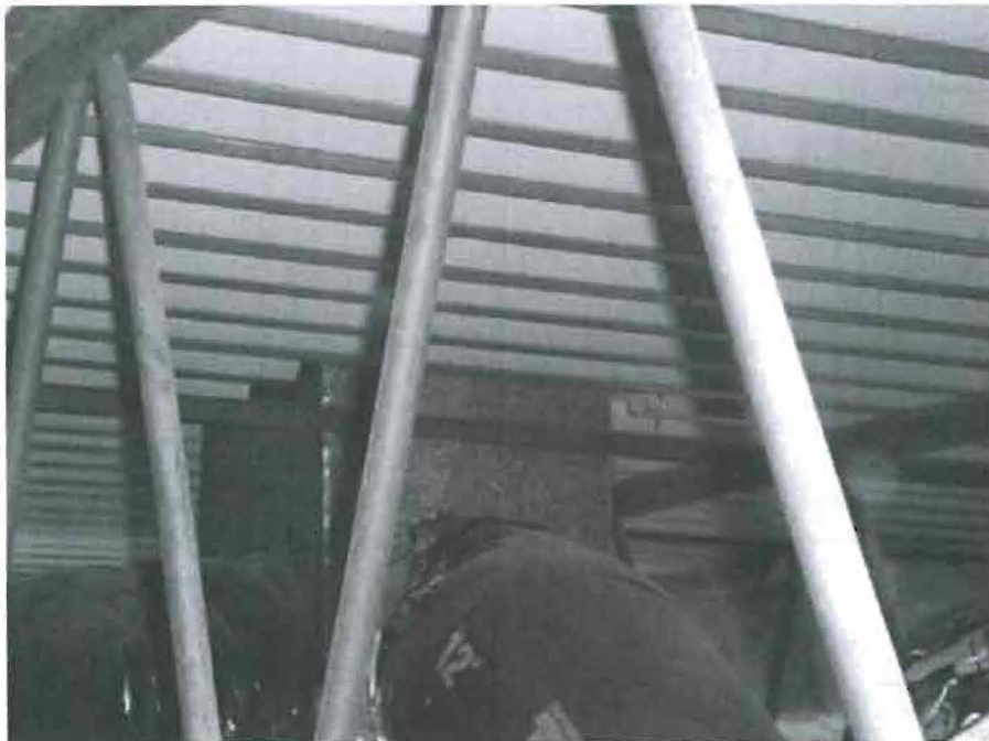
Photo 2: Unreinforced deck penetration at existing duct penetration.
