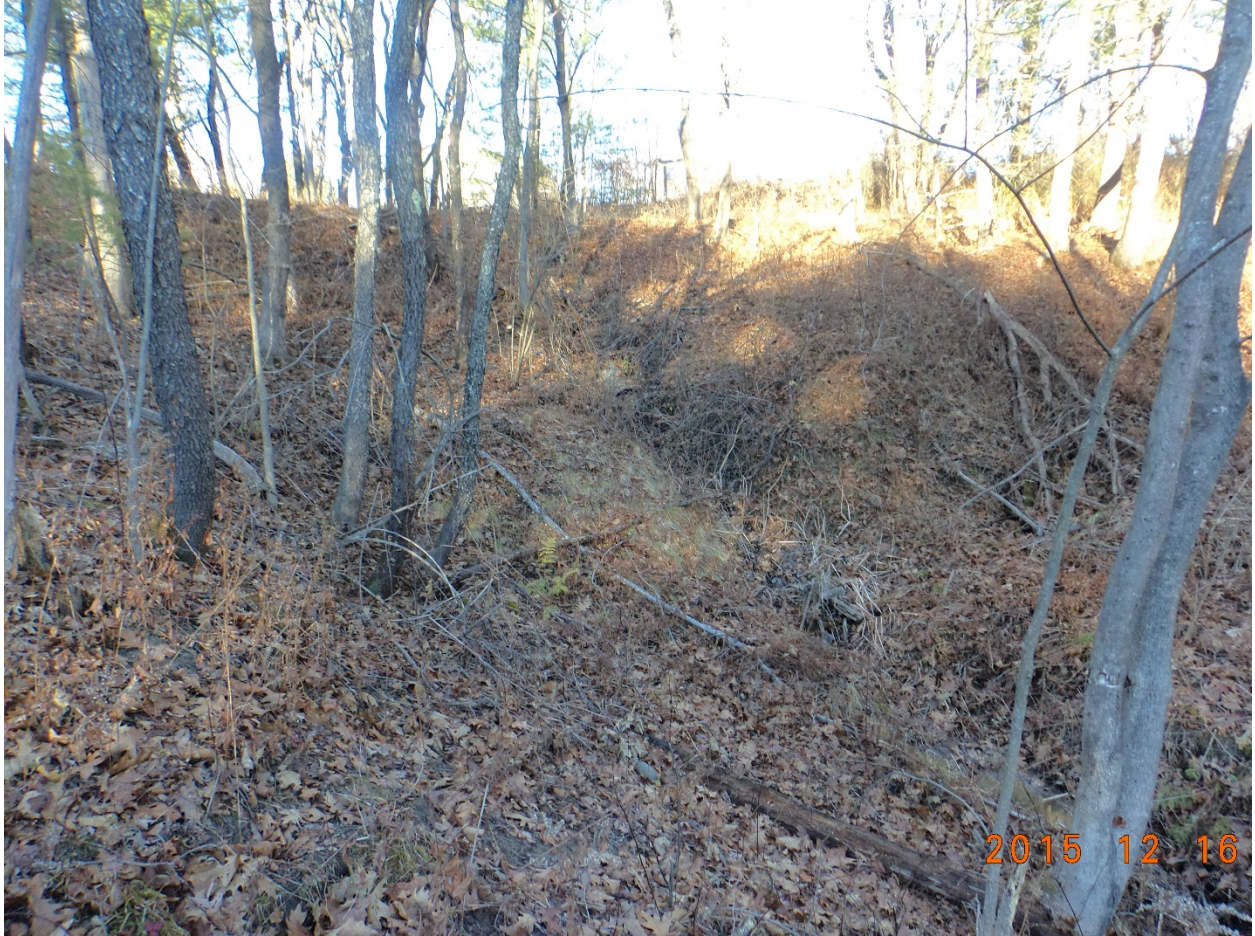
Photo 3: View of existing bank where outfall pipe will extend down. Note slope erosion occurring in the existing condition. New outfall will extend down and outlet at the toe of the slope with velocity reducing rip rap outlet.
