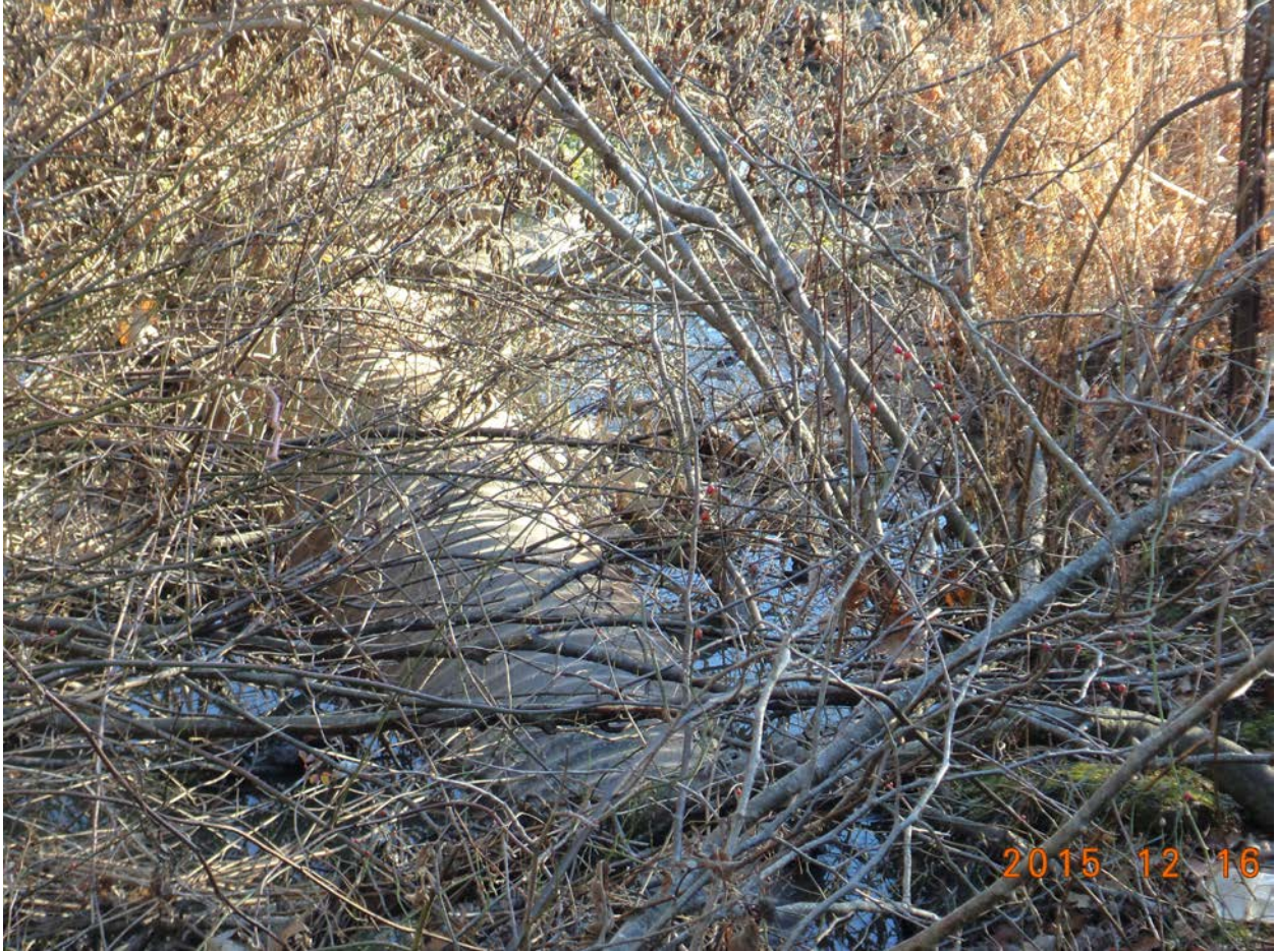
Photo 4: Section of existing CMP culvert that has washed away from the rest of the culvert, highlighting the need for replacement.
