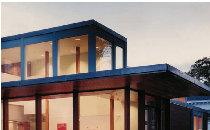
Flashing and trim details should have clean lines and carefully articulated edges. -Waynflete School Arts Center by Scott Simons Architects.
