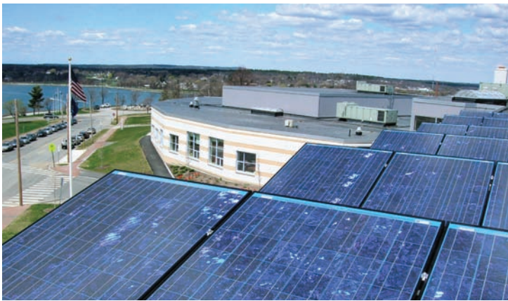
Photovoltaics at Portland's East End School. -Stephen Blatt Architects
