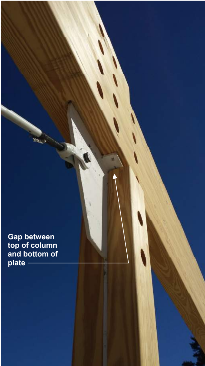
Photo 1: Gaps at Plate Bearing at Braced Frame Columns
