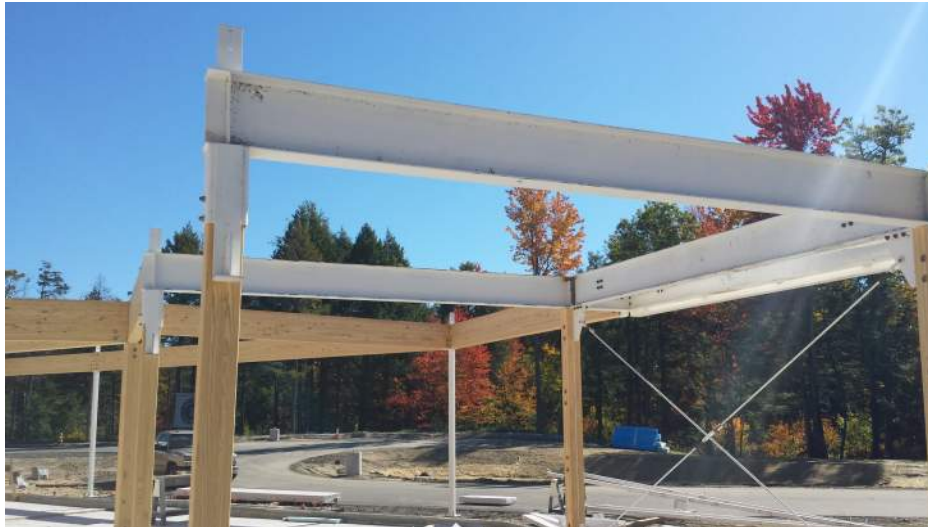
Photo 1: Steel Beam w/o Holes for Web Blocking at Girder Truss Face-Mounted Hanger
