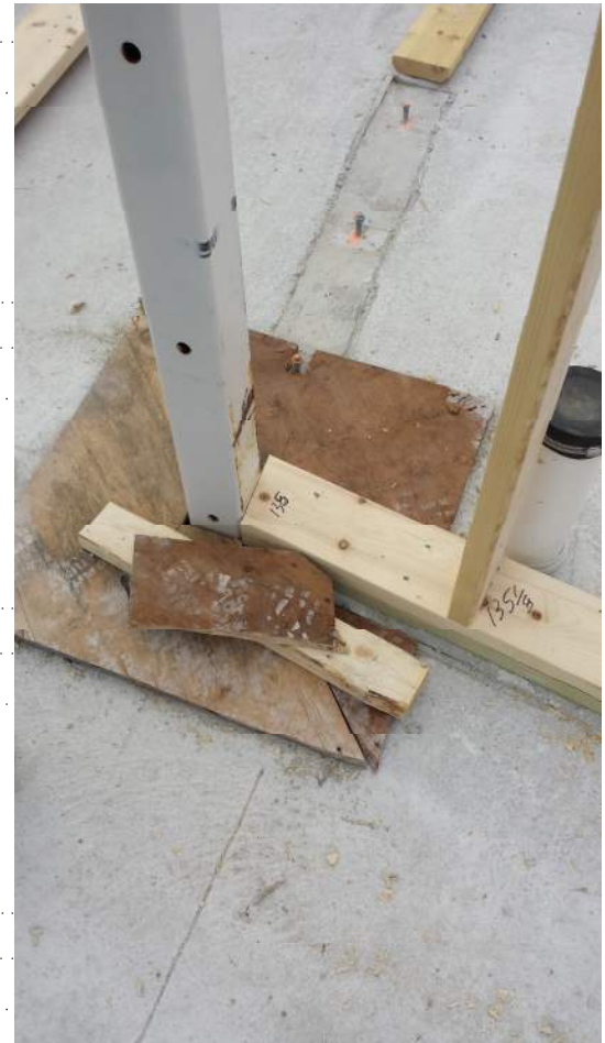
Photo 2: HSS Column w/ Punched Holes on One Face Only
