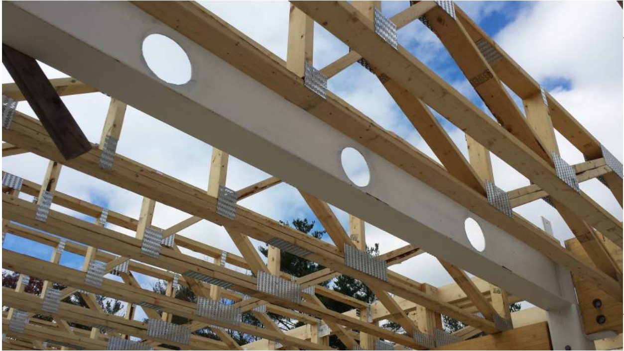
Photo 1: Three Web Penetrations in Steel Beam for New Ductwork
