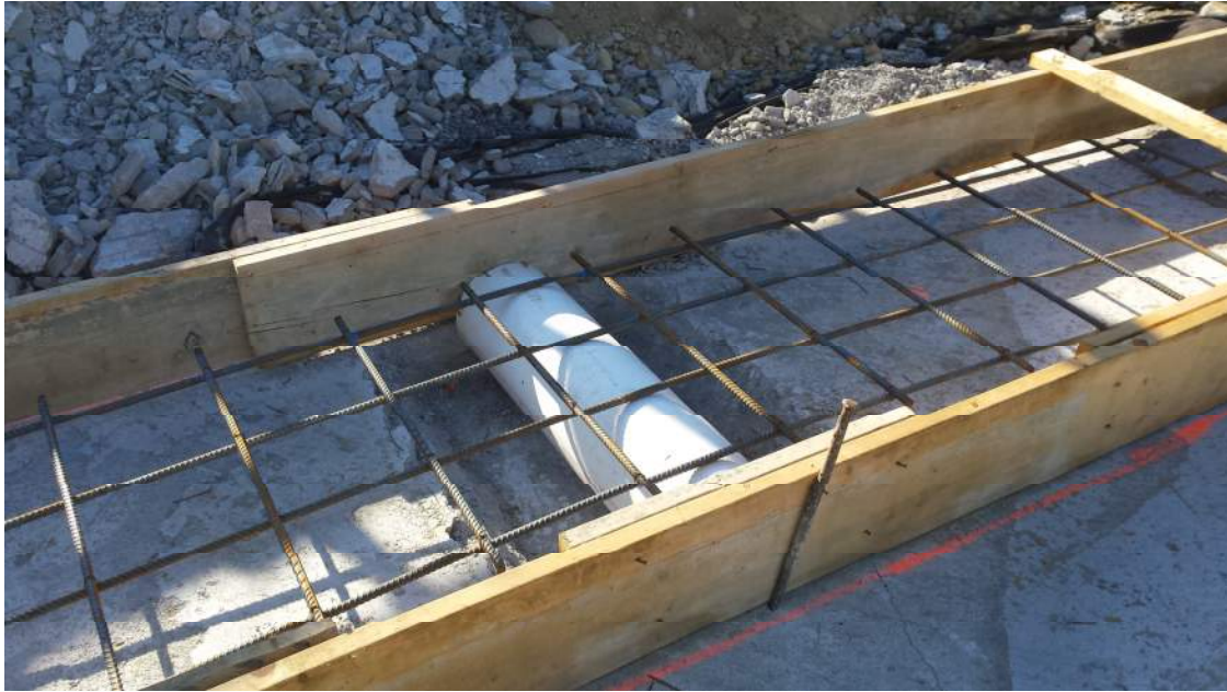
Photo 1: Footing at Pipe Sleeve. Sleeve to raised so that 12" of concrete and reinforcement haunch below pipe.
