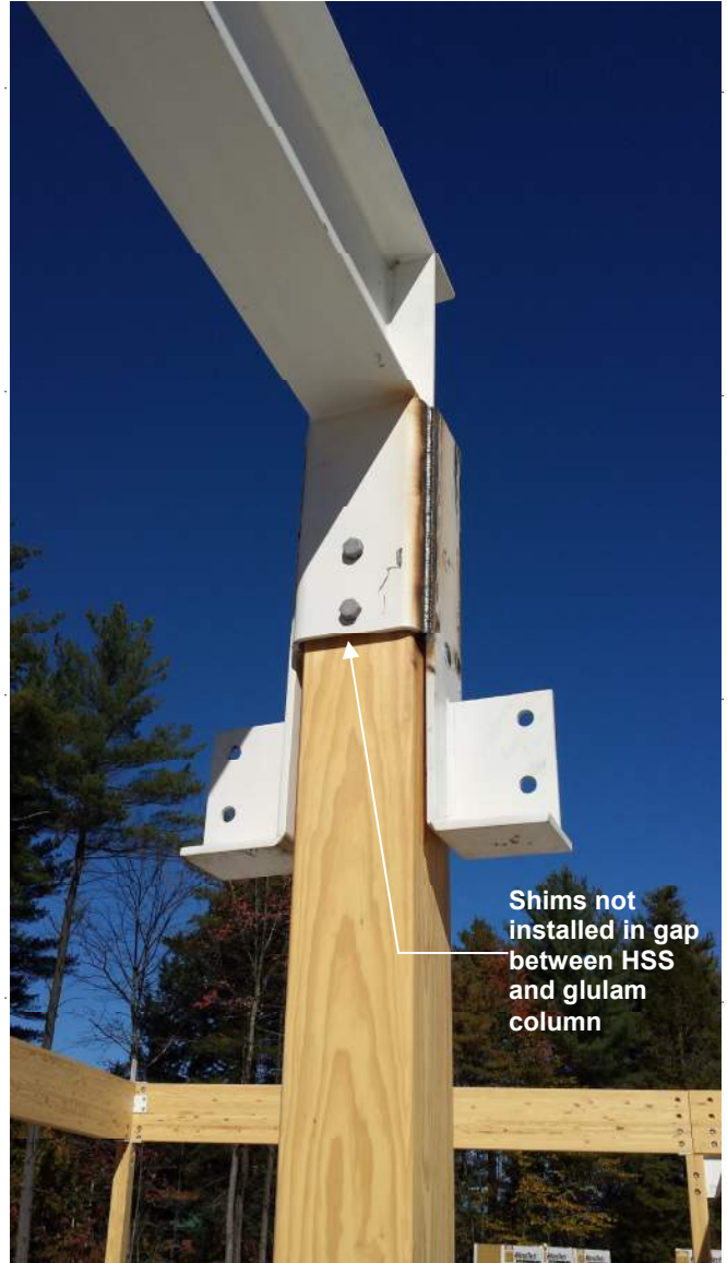
Photo 2: HSS Column Connection w/ Missing Shims
