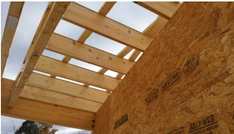
Photo 1: 2x Blocking Between Ladder Framing Not Installed
