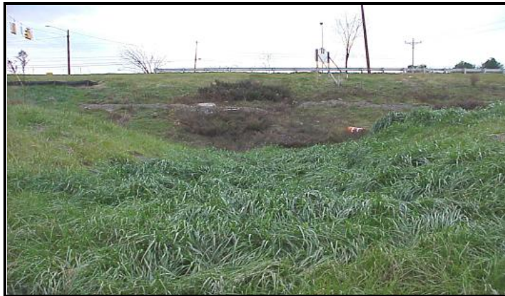
A WELL STABILIZED VEGETATED SWALE SHOWS LITTLE SIGNS OF EROSION VELOCITIES OR FLOWS. THIS SWALE ALSO FUNCTIONS AS A POND SPILLWAY
