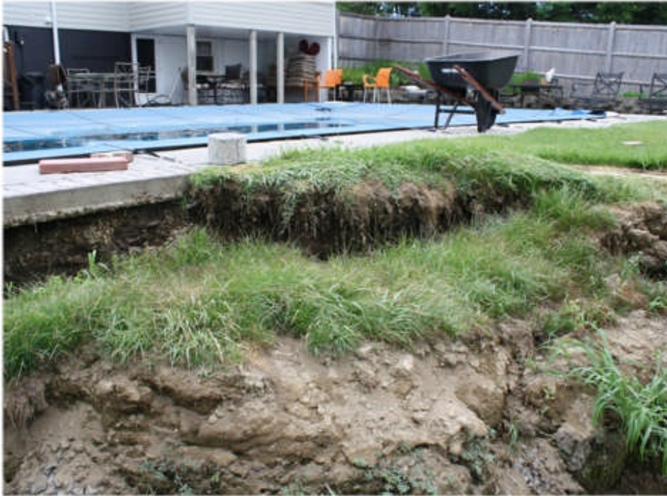
Photo 5. Project Need – Stabilize the slope failure condition (Surface Tension Crack behind house #81)
