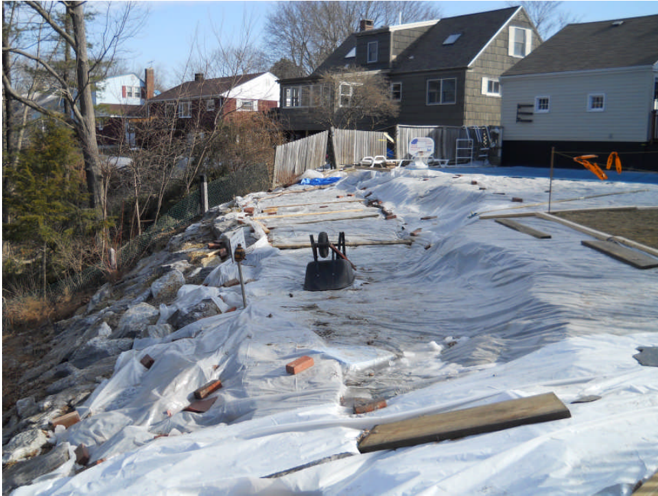
Photo 3. Surface Tension Crack behind house #81
