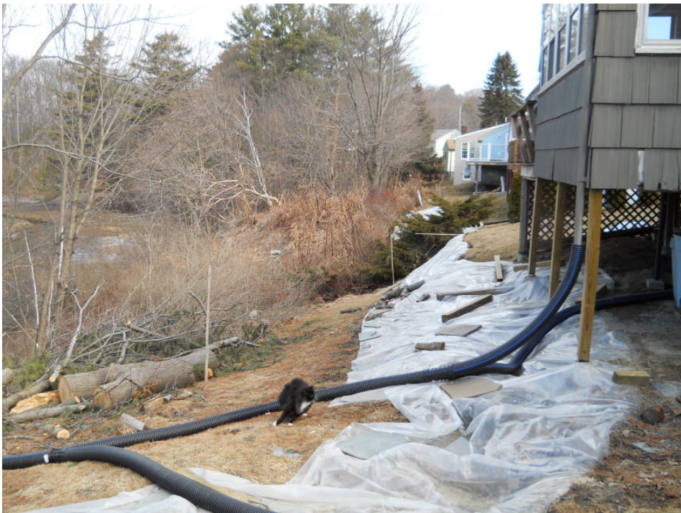
Photo 2. Surface Tension Crack behind house #79
