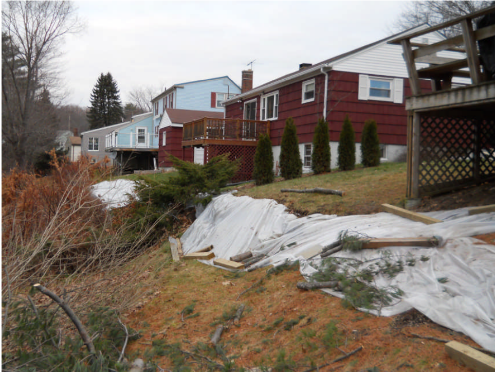
Photo 1. Surface Tension Crack behind house #73
