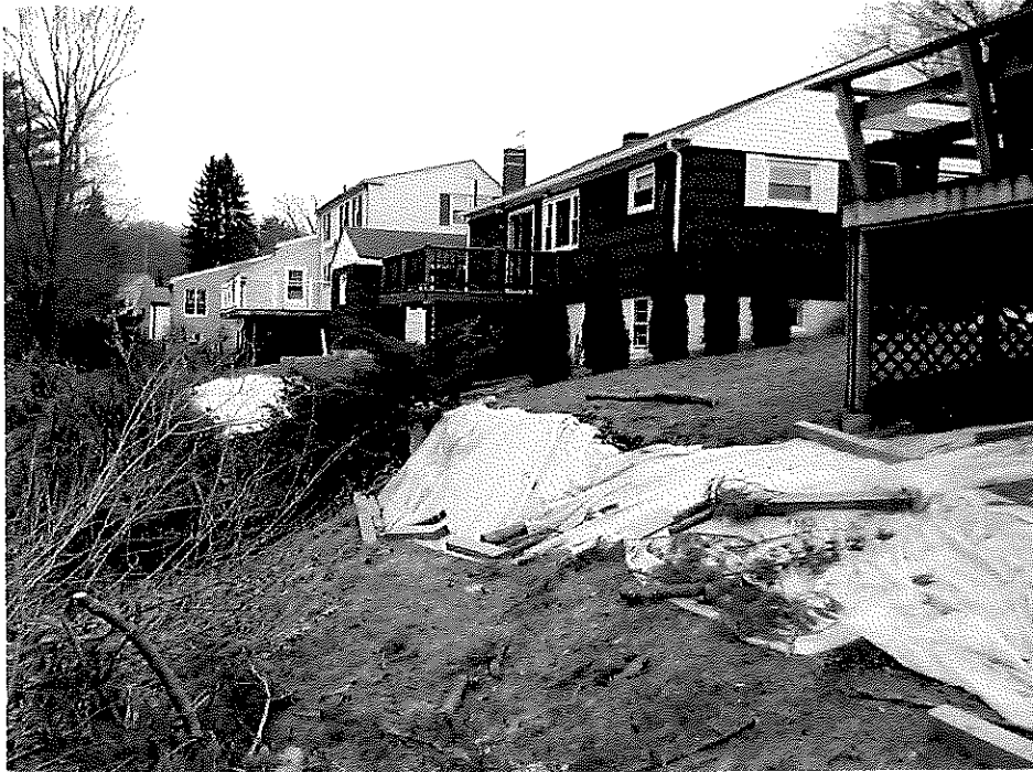
Photo 1. Surface Tension Crack behind house #73
