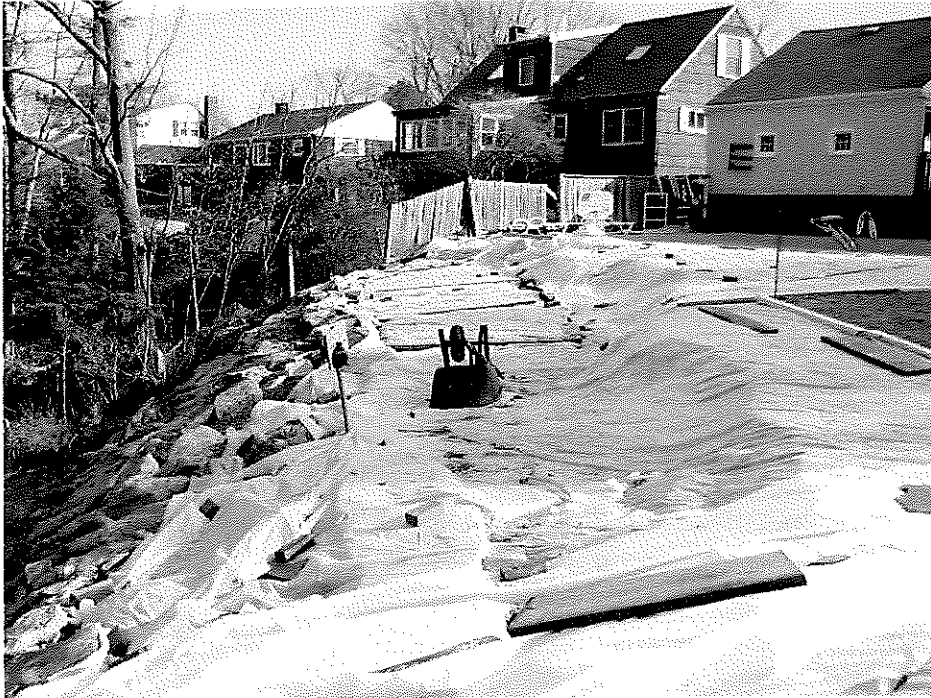
Photo 3. Surface Tension Crack behind house #81
