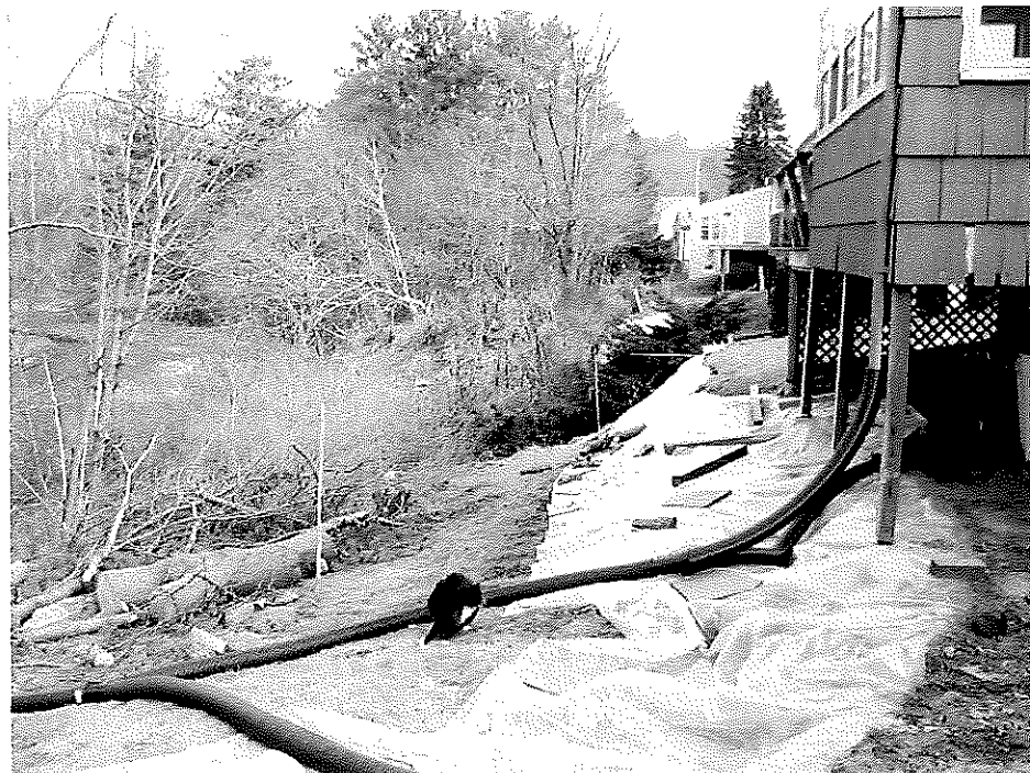
Photo 2. Surface Tension Crack behind house #79
