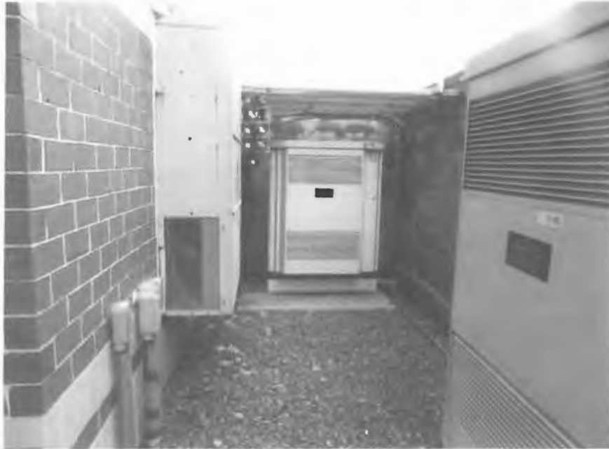
Photo 1: Sample photo illustrating the existing outdoor equipment.
