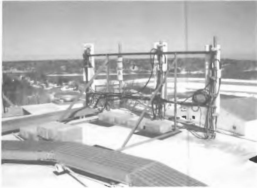
Photo 3: Sample photo illustrating the existing antennas.
