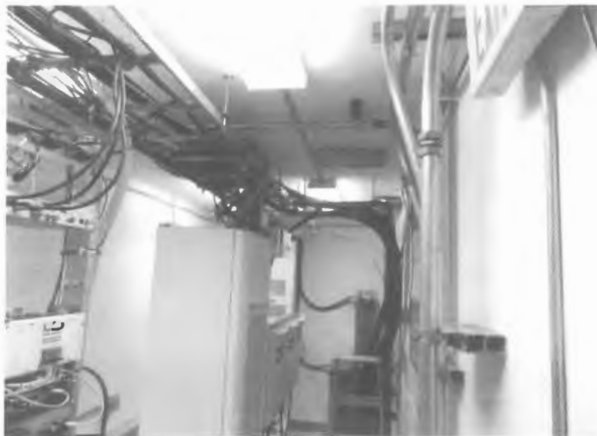
Photo 2: Sample photo illustrating the existing indoor equipment platform
