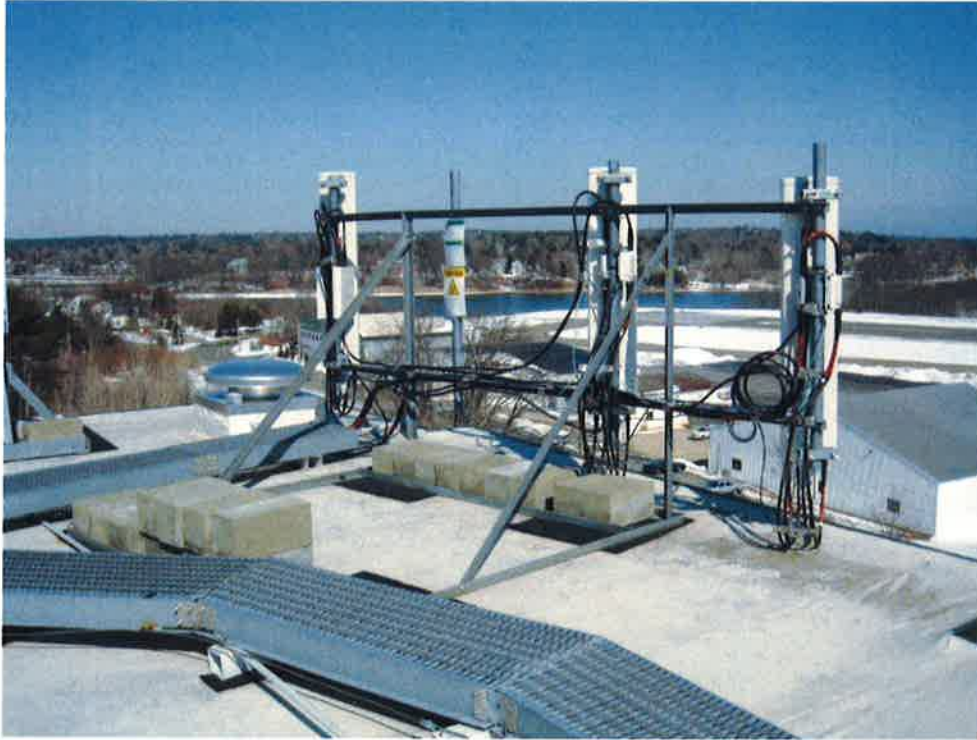
Photo 1: Sample photo illustrating the existing antennas.
