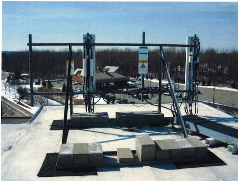
Photo 2: Sample photo illustrating the existing antennas.
