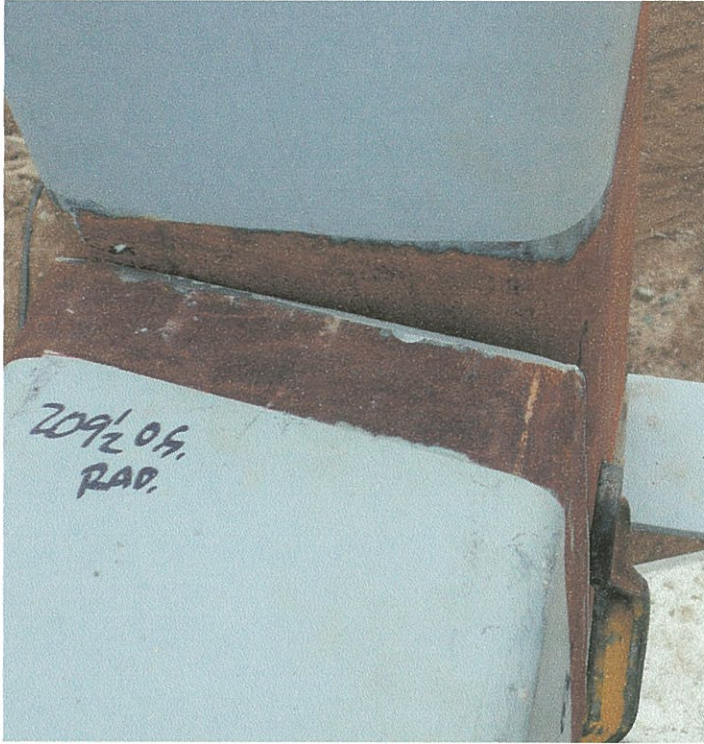
Incorrectly cut HSS beam @ H.3/1 column (side view)
