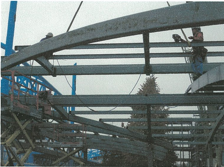
New horizontal tube beams required due to removal of column on grid H.58/13
