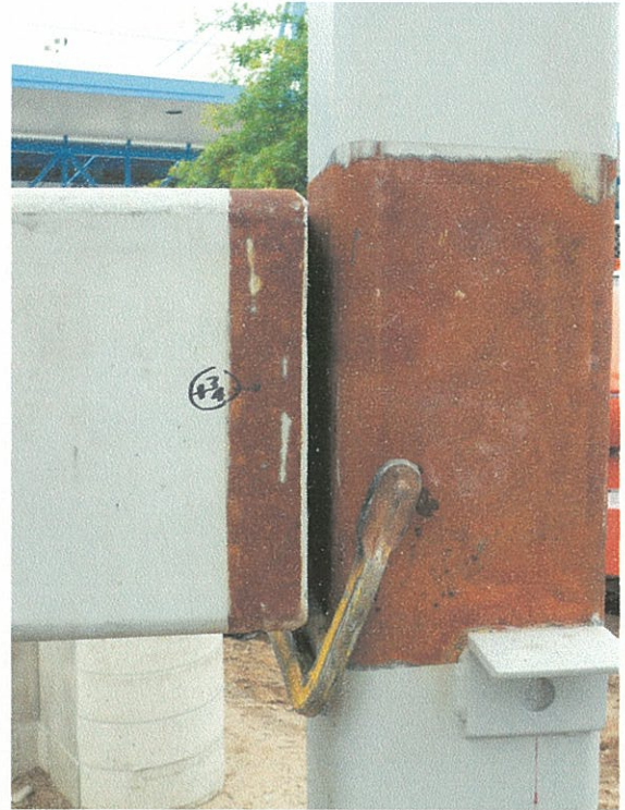
Incorrectly cut HSS beam @ H.3/1 column (side view)
