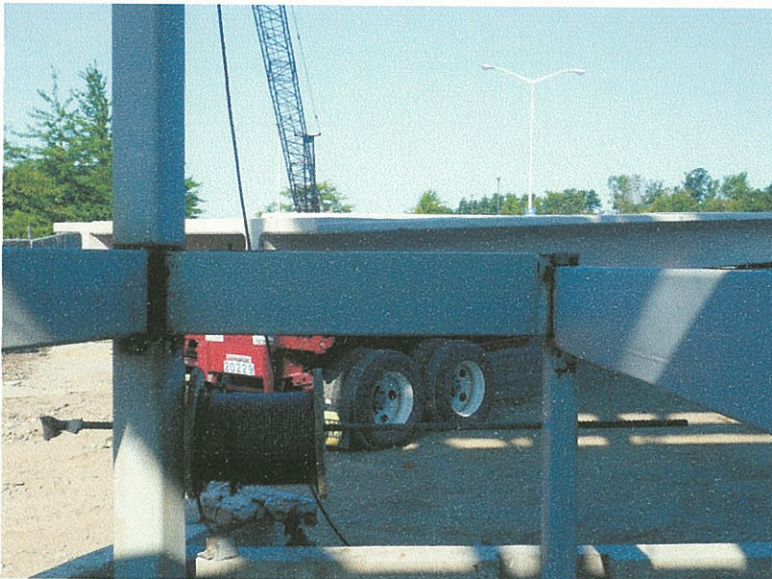
HSS landing beams (center and far left) are raised 2", while HSS flight header (far right) has not been raised.
