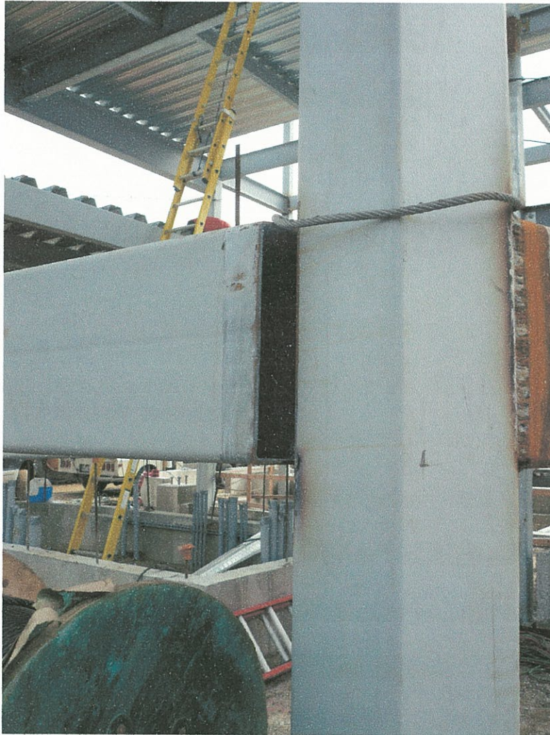
HSS beam incorrectly fabricated, resulting in large opening
