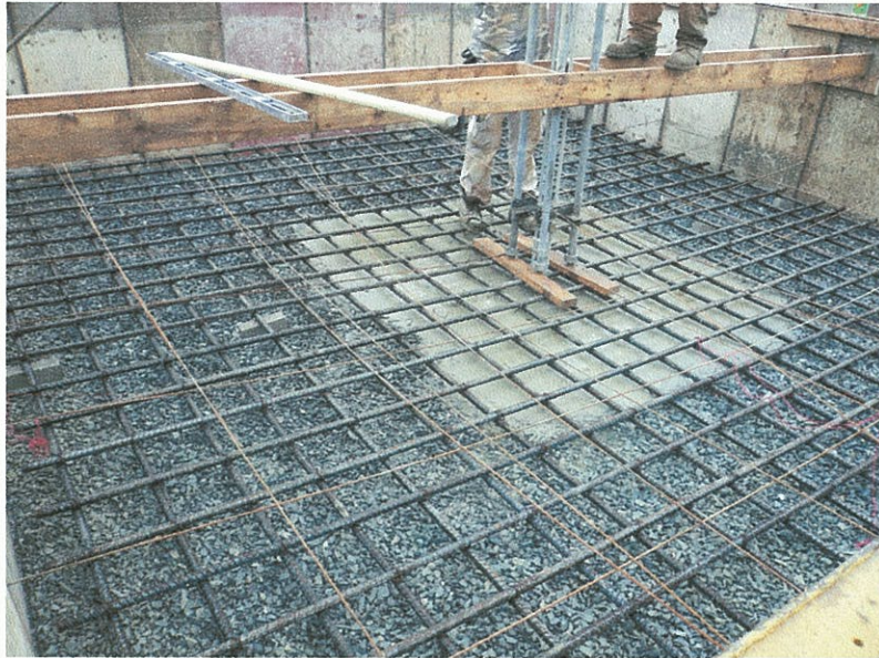
Footing F/2 – Clear cover distance between reinforcement and crushed stone found to be less than the required 3”
