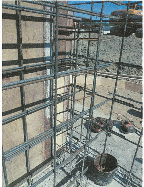
AB's not yet installed
