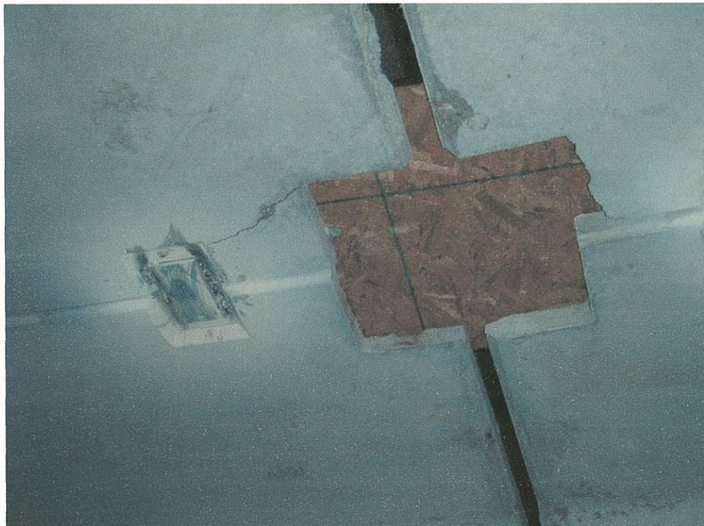
Crack in DT Flange at Drain Blockout
