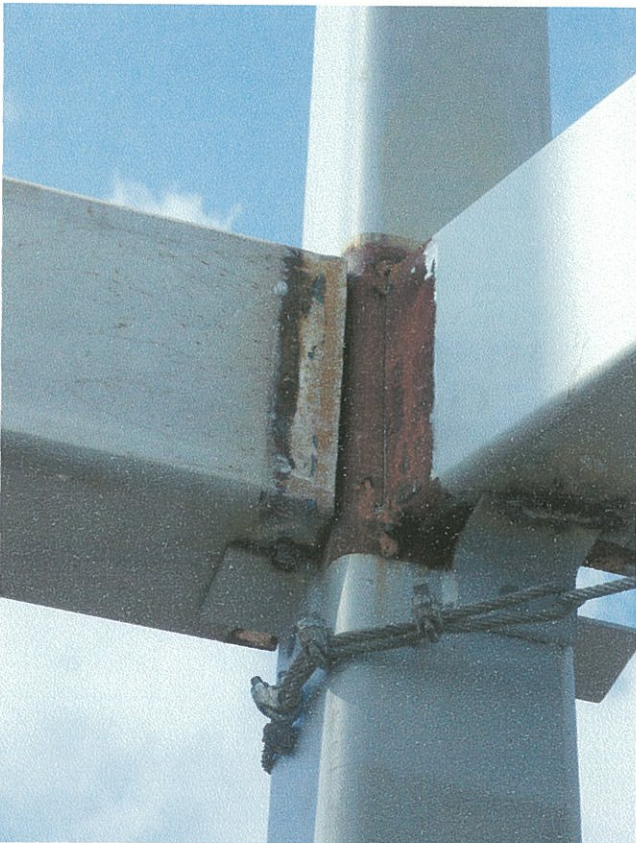
3" Tube stub (left) full pen welded to beam @ Grid 1 (view from inside Stair Tower)
