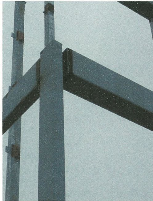
HSS landing beam cut short of column
