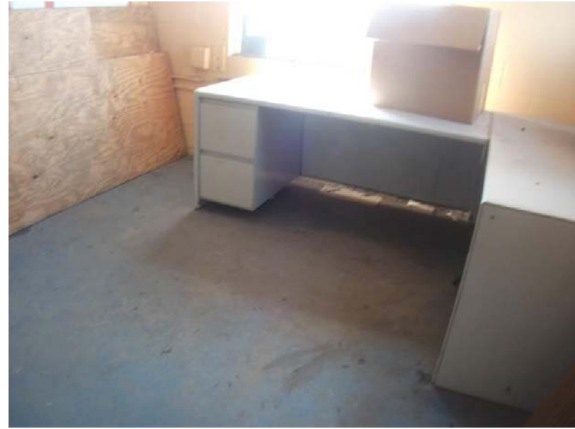
2. Potential lead and PCB paint on floors in Building #3.
