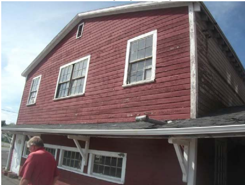
7. Potential lead and PCB paint on walls and trim, potential ACM window glazing, on exterior of Building #2.
