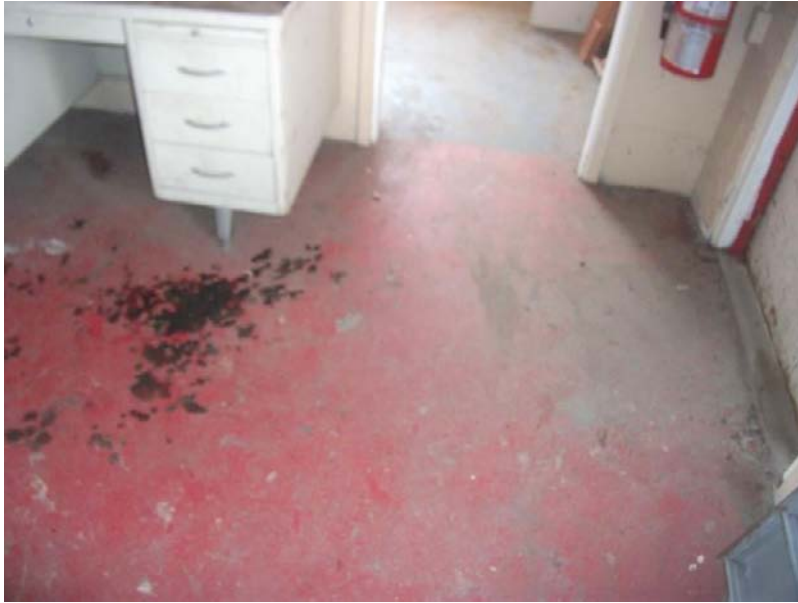
1. Potential lead and PCB paint on floors in Building #3.
