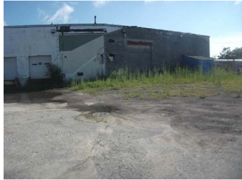
10. Potential lead and PCB paint on walls on exterior of Building #5.
