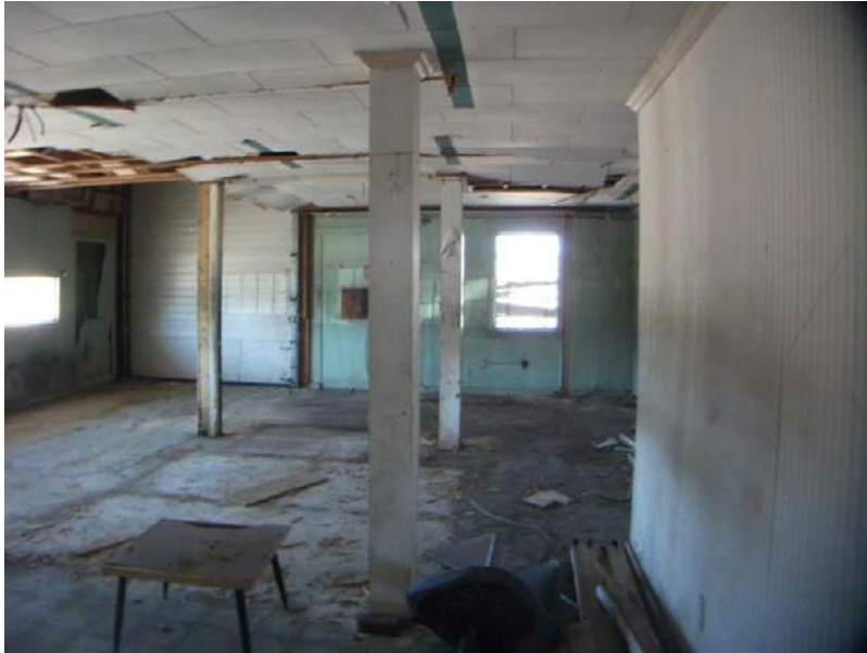
5. Potential lead and PCB paint on walls and floors, potential ACM floor tile, and waste fluorescent lighting in Building #2, room 1.
