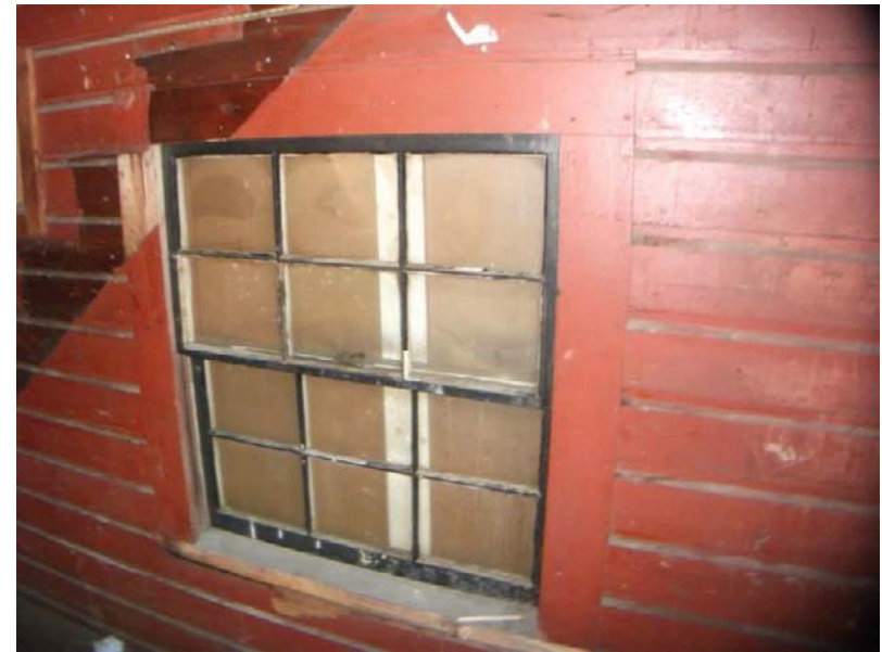
8. Potential lead and PCB paint on walls and potential ACM window glazing in Building #2, room 2.
