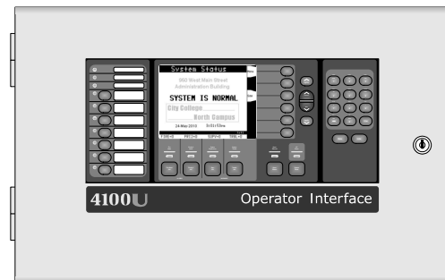
InfoAlarm Command Center in Remote Cabinet
