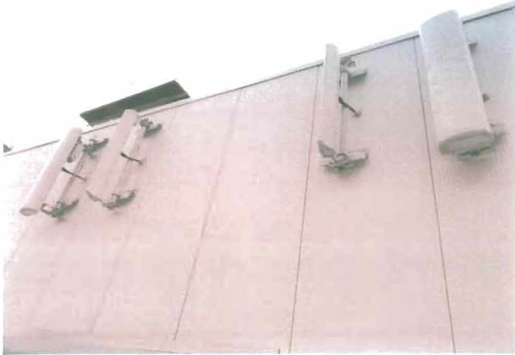
Photo 1: Sample photo of the existing Verizon Antennas secured to the penthouse wall.
