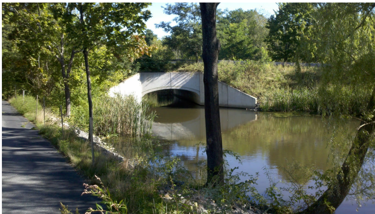
Figure 4-3 View of culvert crossing under Capisic Street, facing northeast (Photo by Woodard & Curran, September 2012)
