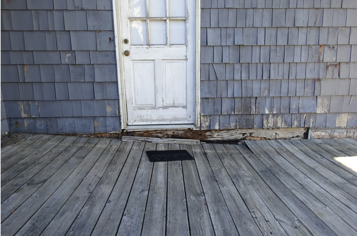
Photo 2. Closer view of collapsed area at center of deck. The door will be removed, the opening filled in (framed, sheathed) and finished with wood shingles matching the existing. 11 Stevens Avenue, Portland, ME. Photo taken April 30, 2016.
