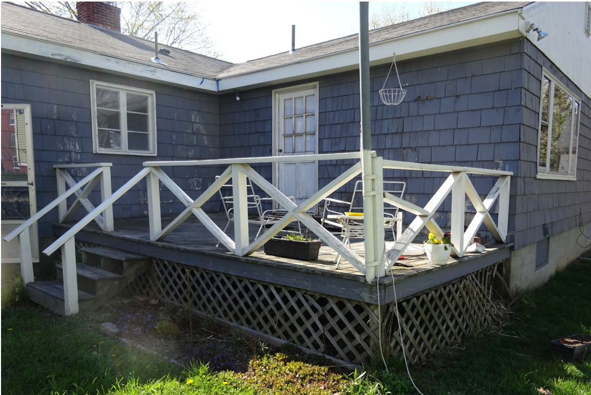
Photo 1. Deck, steps to deck, and door to house, all to be removed. 11 Stevens Avenue, Portland, ME. Photo taken April 30, 2016.
