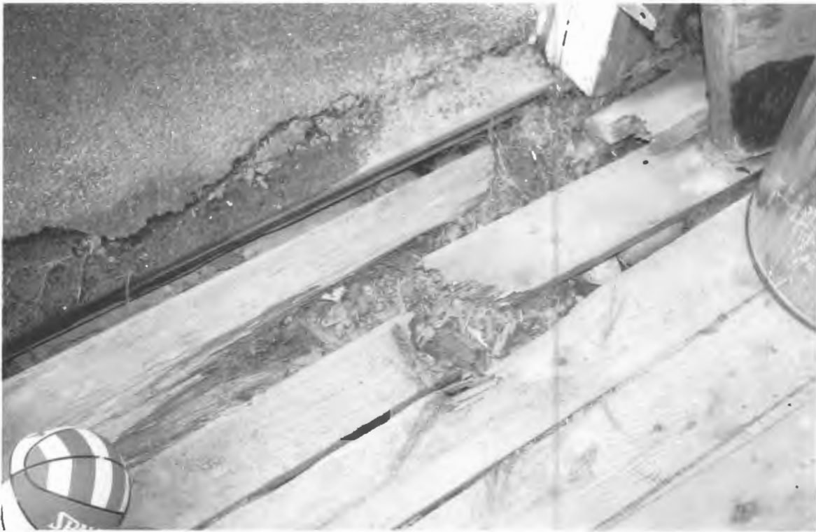
Existing garage floor to be replaced.
