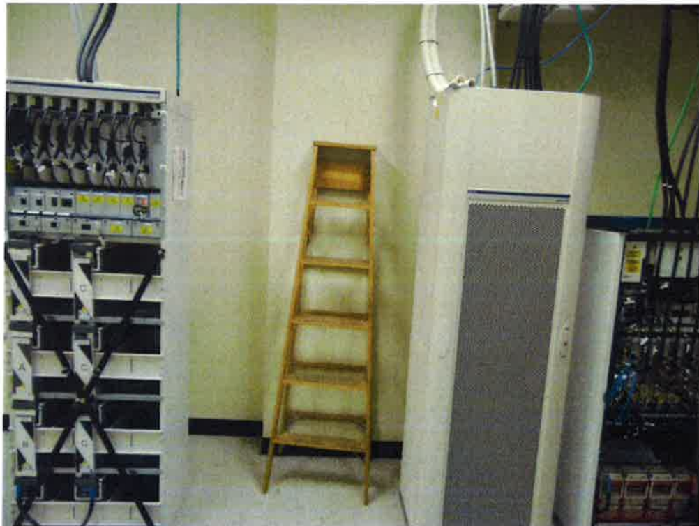
Photo 4: Sample photo showing the existing T-Mobile equipment.
