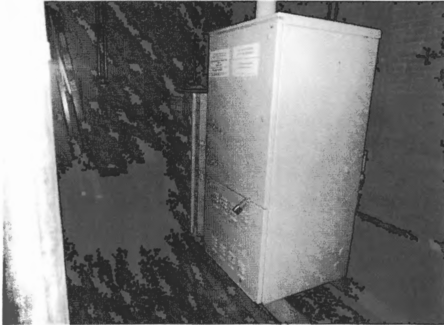
Photo 4: Sample photo showing the existing Sprint equipment platform.
