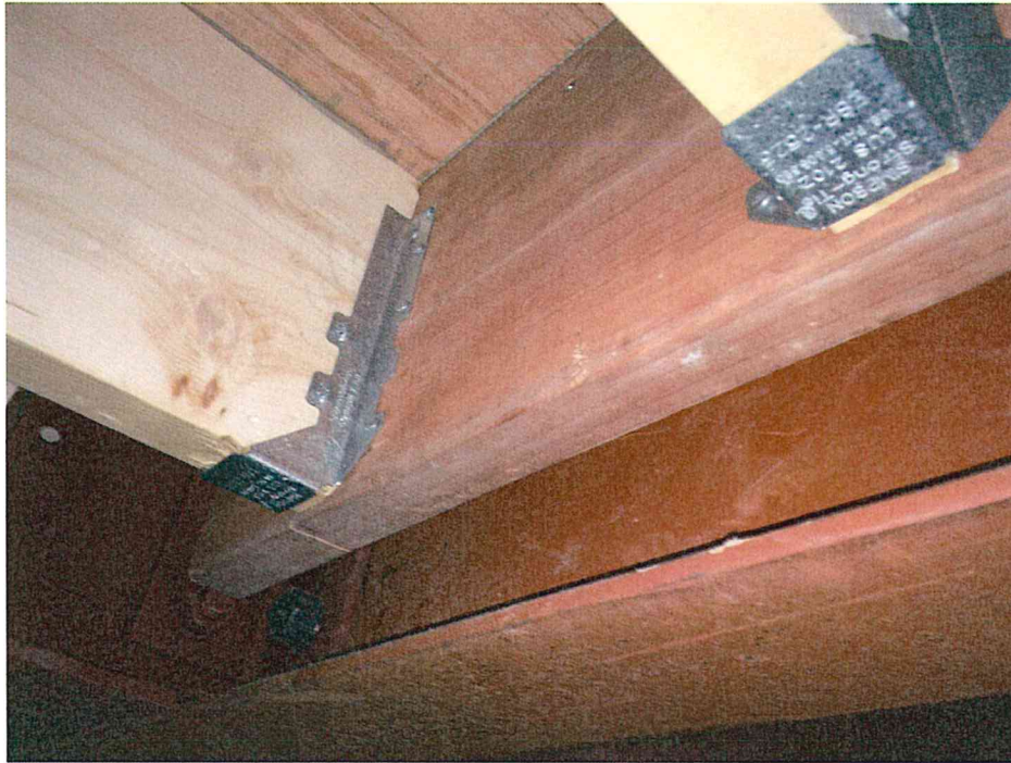
Photo # 1 -Infill joists running the wrong direction and ledger inadequately fastened to existing beam.
