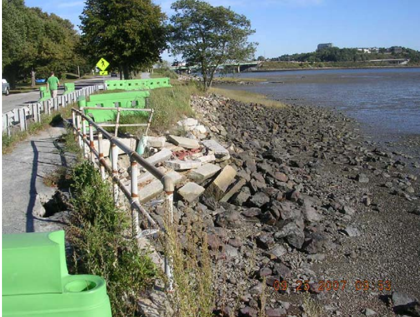
Figure 1. The damaged trail adjacent to the retaining wall (2007-09-26)
