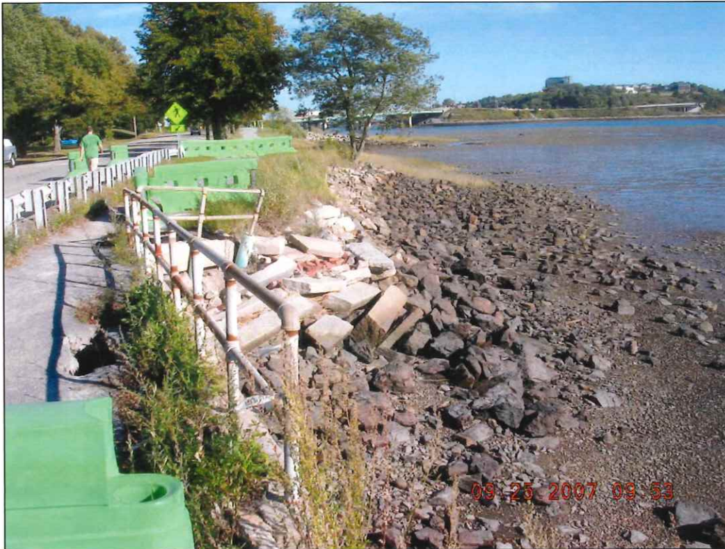
Photo 1: The damaged trail adjacent to the retaining wall (2007-09-26).
