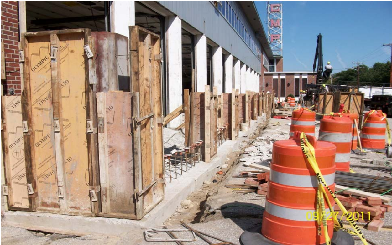
09-27-11 Wall and pier forming and reinforcing for new addition walls and piers.
