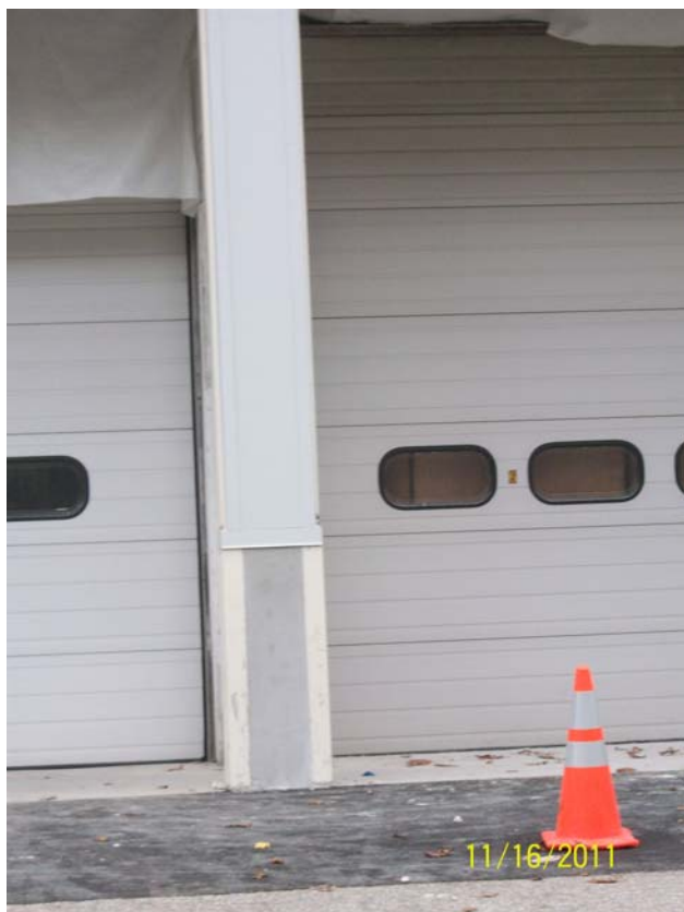
11-16-11 an example of one of the piers after the concrete was coated with SILPRO.
