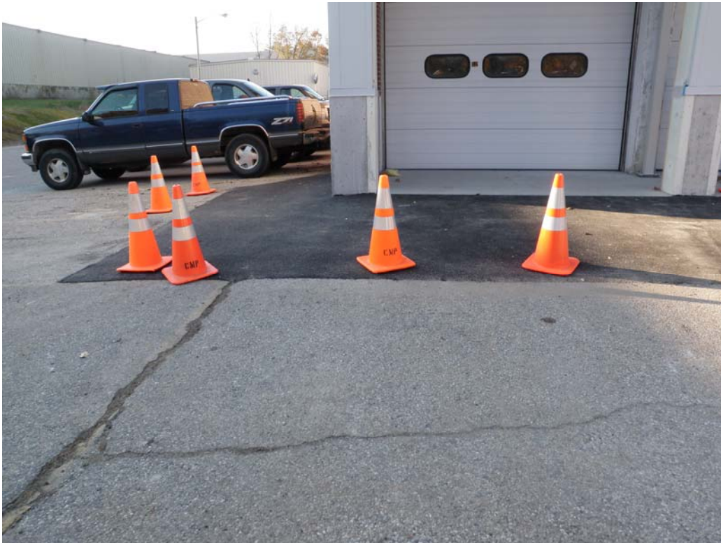
11-09-11 area of pavement to be removed & repaired.
