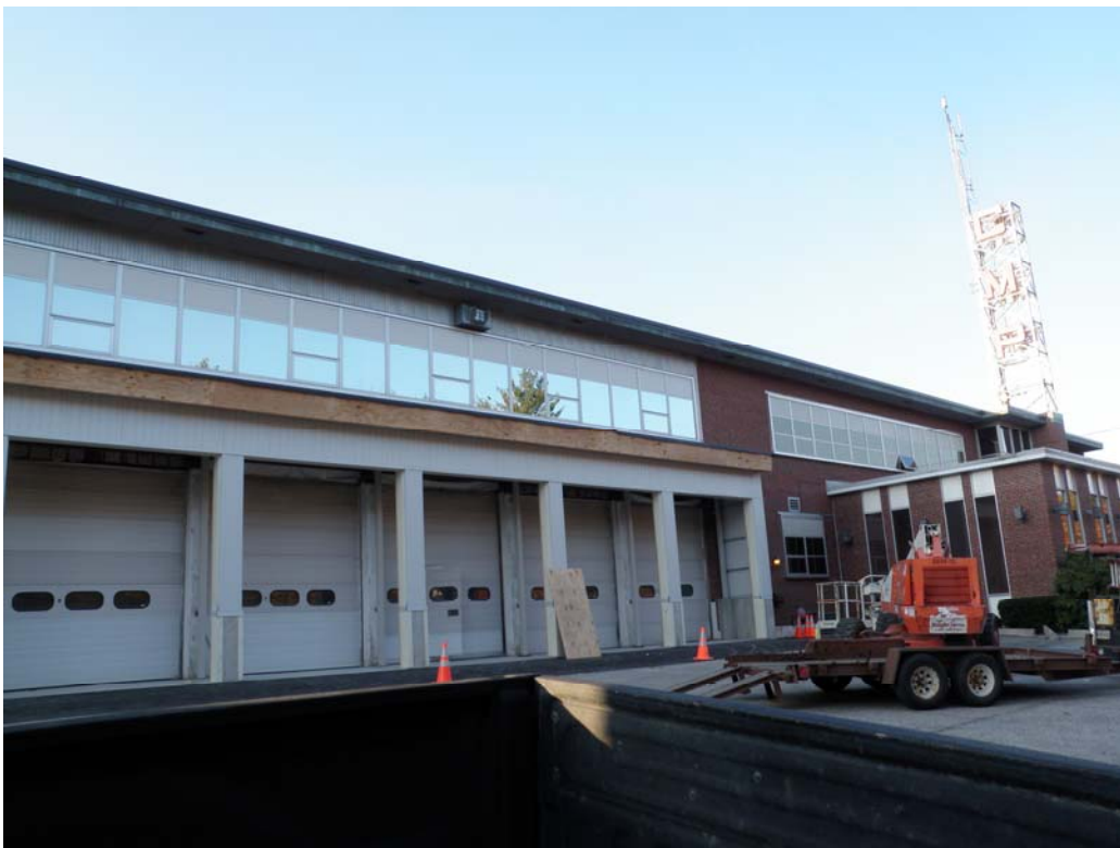
11-09-11 all of the siding is on and the roof membrane is glued down no aluminum fascia on this section.
