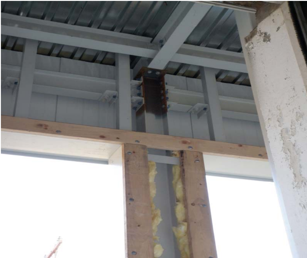
11-09-11 door bucks and insulation installed between overhead doors, plywood is cut and waiting to be painted.
