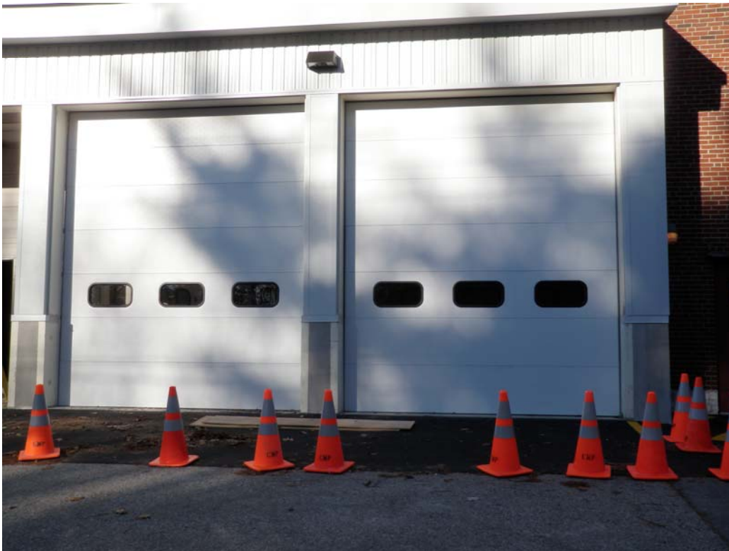
12-02-11 exterior new overhead doors assembled & stacked. Also, Wiswell Electric has installed the exterior wall mount lights between every other door.
