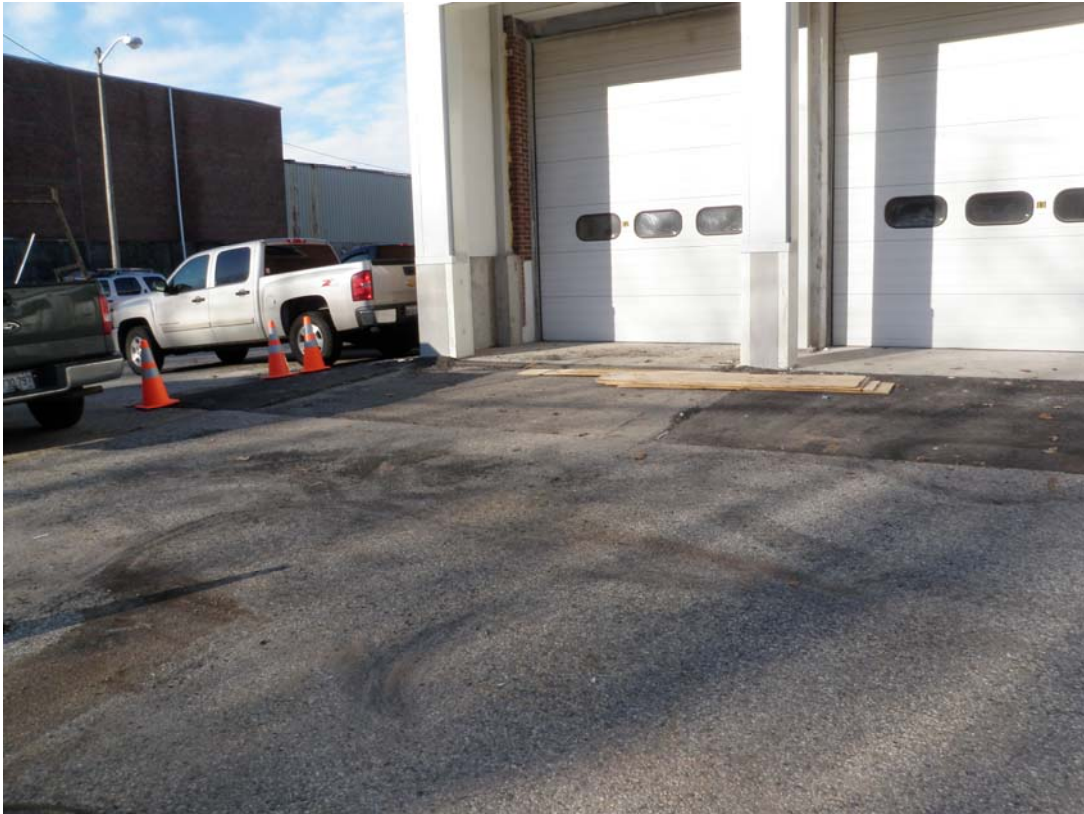
12-02-11 repair area has been ground out waiting on new wearing course to be installed.
